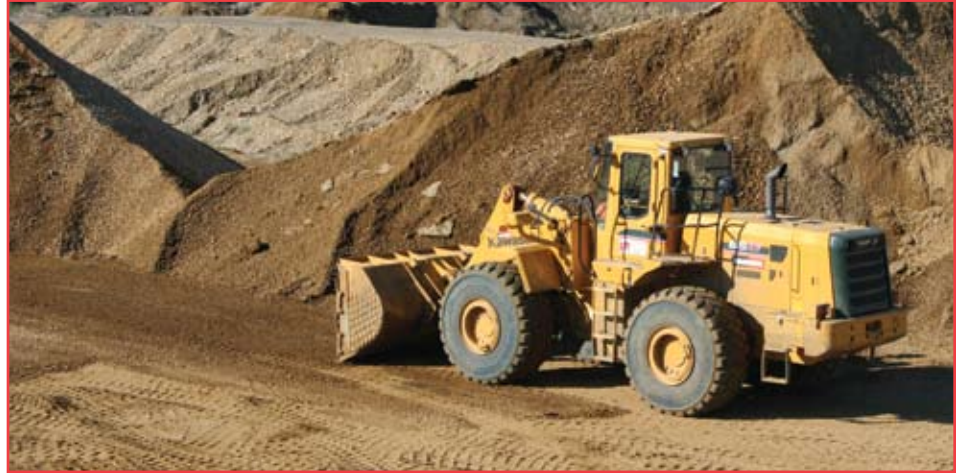
The well-balanced aspect of the Kawasaki loader, coupled with careful pad maintenance, eliminates rutting. Despite the abrasive nature of the material, the loader backdrags without resistance.
